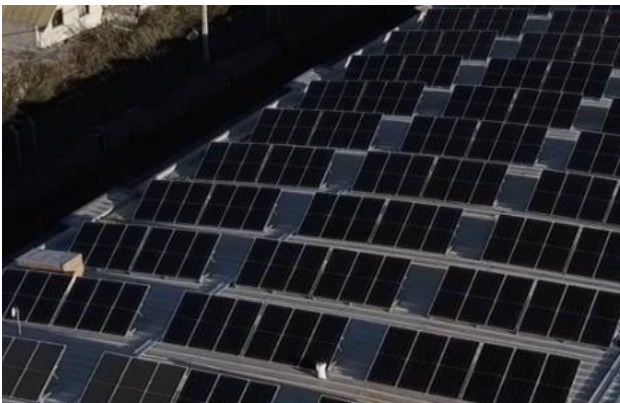
Figure 1: PV modules aligned to the south
